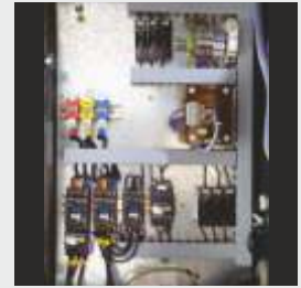
Electrical Cubicle Monitors Power Management
